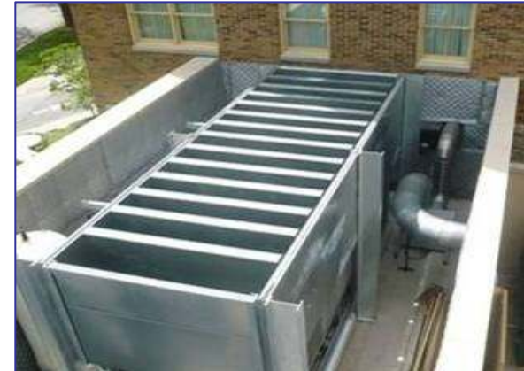
Silenced Discharge Stacks
